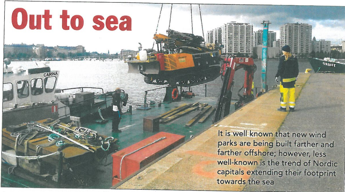
A Geomachine GM100 drill rig is lifted onto a barge by the Helsinki Geotechnical Department for sea-bottom investigation for a bridge link from east Helsinki to the downtown area
