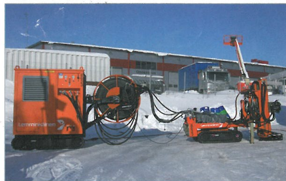
The first two GM-Kelpo units are in operation under the main railway station in Stockholm, Sweden
